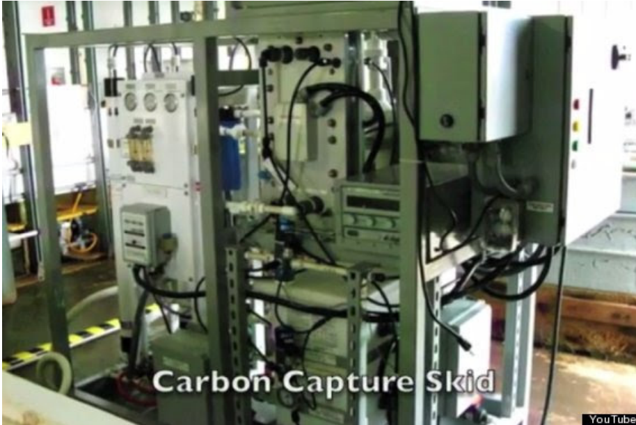
The carbon-capture system developed by the NRL
